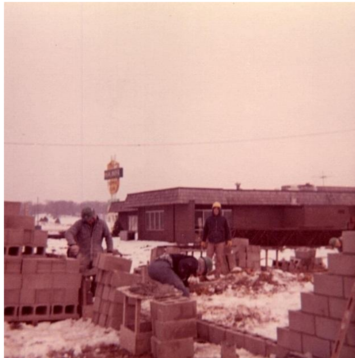
Figures 8-40, 8-41: Construction photos; Left, looking west, supper club and sign, note footings and new south entry, right, supper club original north wall looking southwest, both December 1972 (Courtesy of Sheila Boyd)
