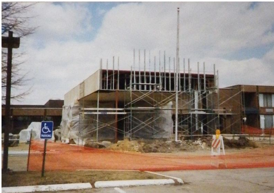
Figure 8-118: Radisson remodeling of the south portico, 1997, looking northeast (Courtesy of Sheila Boyd)
