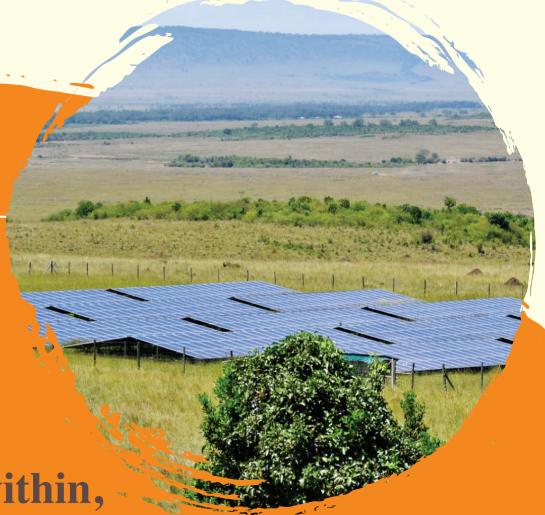
Solar Plant Tour
