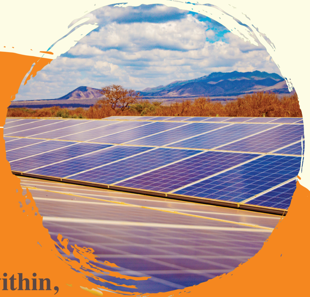
Solar Plant Tour
